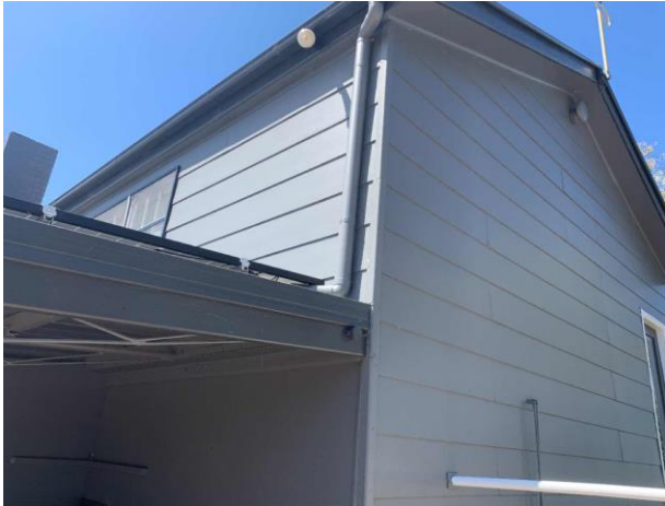
Line ID 42: External, Old Recreation Hall, All Elevations, Wall Cladding, Fibre Cement Sheet - Chrysotile, Amosite and Crocidolite Asbestos Detected
