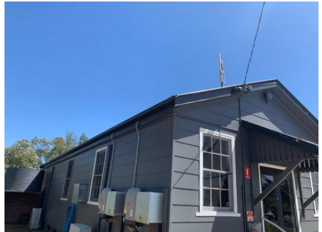
Line ID 20: External, Hilltop Lodge, Elevations, Weatherboard Cladding and Joinery, Fibre Cement Sheet - Chrysotile & Amosite Asbestos Detected
