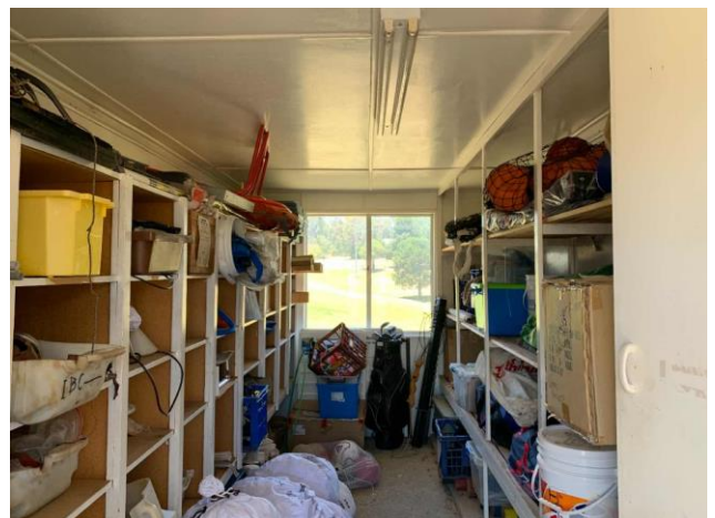
Line ID 162: Internal, Workshop, Basement Store, Fluorescent Lights, Capacitor(s) - Suspected PCB
