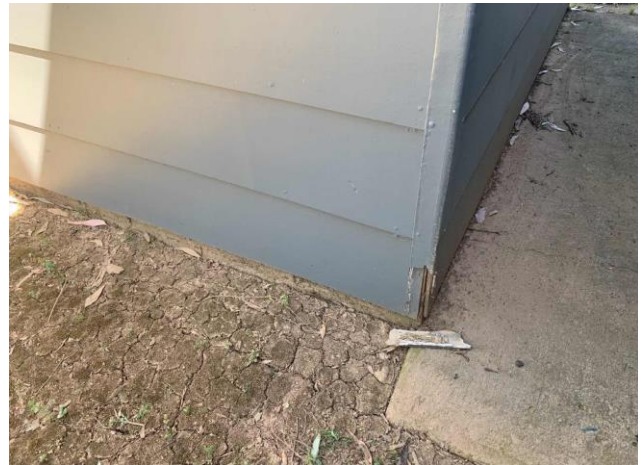
Line ID 8: External, Bike Shed (Formerly Male Toilet Block), Guest Shower/Toilet Block, Weatherboard Cladding and Joint Cover Strips, Fibre Cement Sheet - Chrysotile & Amosite Asbestos Detected
