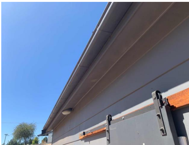
Line ID 10: External, Bike Shed (Formerly Male Toilet Block), Throughout, Eaves Lining, Fibre Cement Sheet - Chrysotile Asbestos Detected
