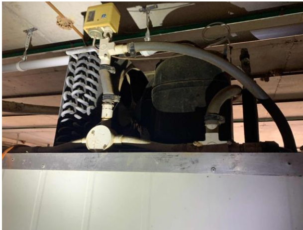
Line ID 168: Internal, Dining Hall, Basement, Refrigeration Unit, Unknown Refrigerant - Suspected ODS
