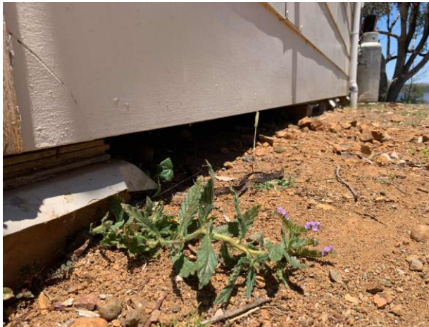
Line ID 28: External, Kilpara, Subfloor, Column Packers, Fibre Cement Sheet - Chrysotile, Amosite and Crocidolite Asbestos Detected
