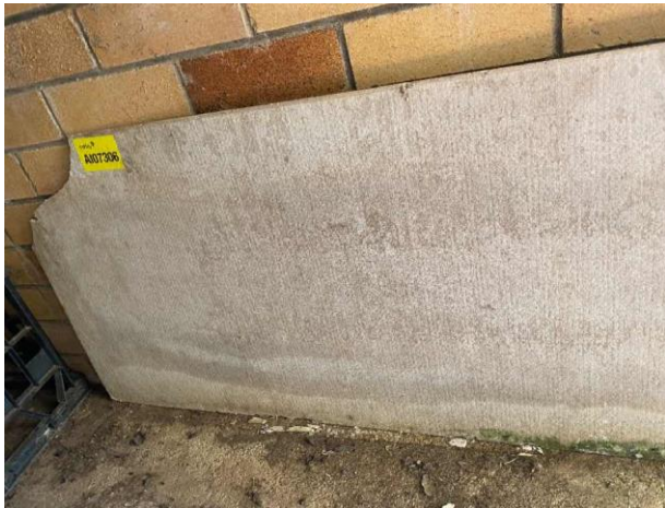
Line ID 48: External, Private Residence A, Backyard, Under Water Tank in Brick Housing, Stored Fibre Cement Sheet - No Asbestos Detected
