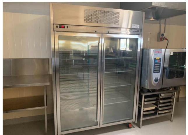
Line ID 171: Internal, Homestead, Throughout, Kitchen, Fridge, Unknown Refrigerant - Suspected ODS
