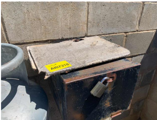
Line ID 90: Internal, Liquid Gas UST Enclosure, Within Enclosure, on Lockbox and Signage Placards, Debris, Compressed Cement Sheet - Chrysotile Asbestos Detected
