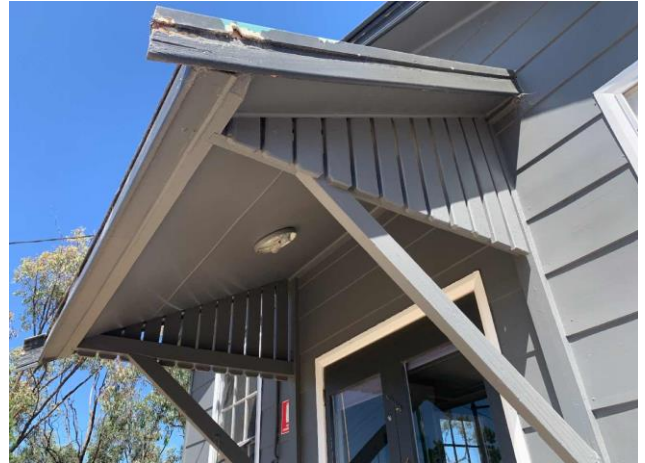
Line ID 43: External, Old Recreation Hall, Facades, Weatherboard Cladding and Joinery, Fibre Cement Sheet - Chrysotile & Amosite Asbestos Detected
