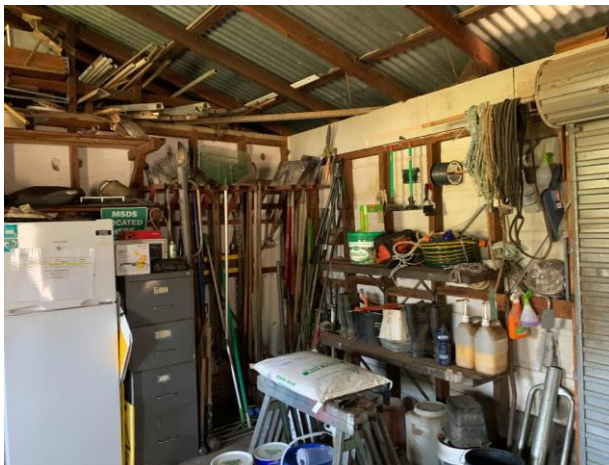
Line ID 115: Internal, Workshop, Between Workshops, North Wall Partition, Fibre Cement Sheet - Chrysotile Asbestos Detected
