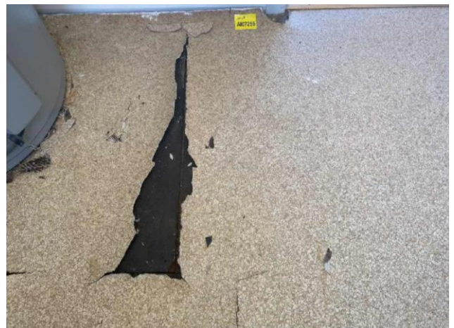
Line ID 110: Internal, Staff Quarters and Accommodation, Cleaners Storage Room, Floor Covering, Paper Backed Beige Vinyl Sheet with Attached Bituminous Material - Chrysotile Asbestos Detected
