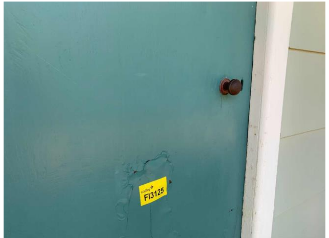
Line ID 126: External, Hilltop Lodge, Elevations, Doors Throughout, Green-Blue Paint - Lead Detected (<0.005% w/w)
