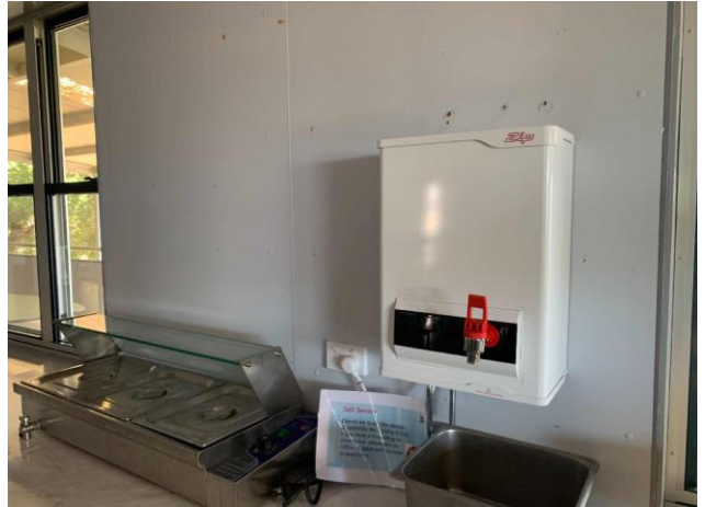
Line ID 152: Internal, Dining Hall, Throughout, Kitchenette, Boiler Above Sink, Internal Insulation - Suspected SMF
