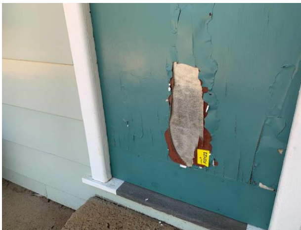
Line ID 127: External, Hilltop Lodge, Elevations, Doors, Lower Layer Paint, Brown Paint - Lead Detected (0.01% w/w)
