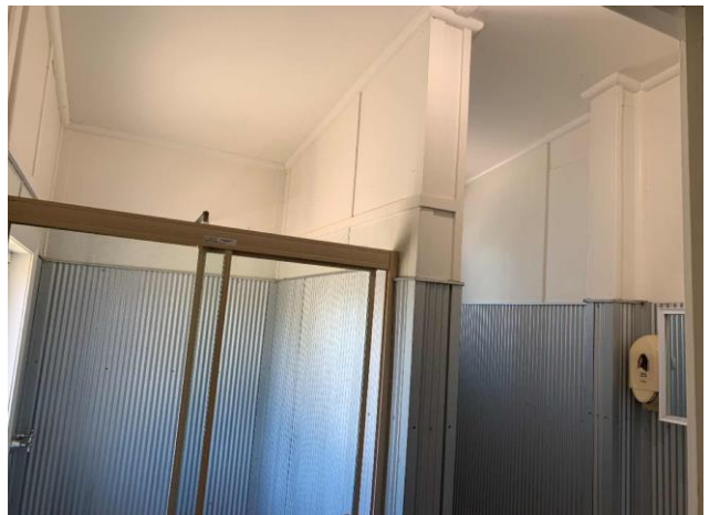
Line ID 89: Internal, Kilpara, Toilets and Shower, Walls and Ceiling Lining, Fibre Cement Sheet - Chrysotile Asbestos Detected
