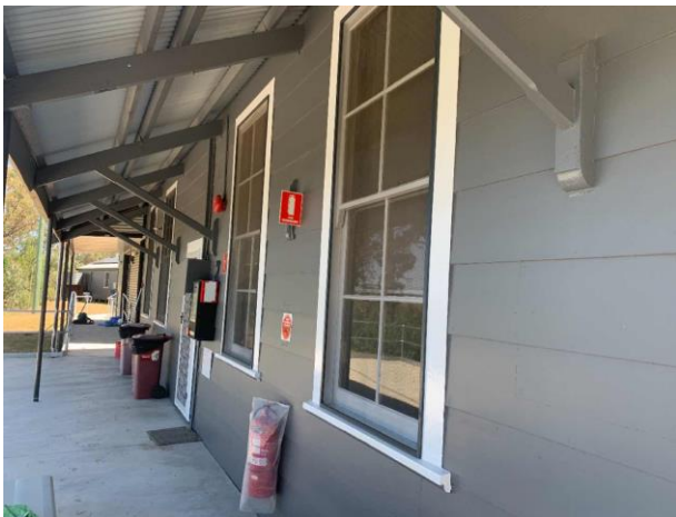
Line ID 40: External, Old (South) Dormitory, East and West Face, Cladding Barge Boards, Fibre Cement Sheet - Chrysotile & Amosite Asbestos Detected
