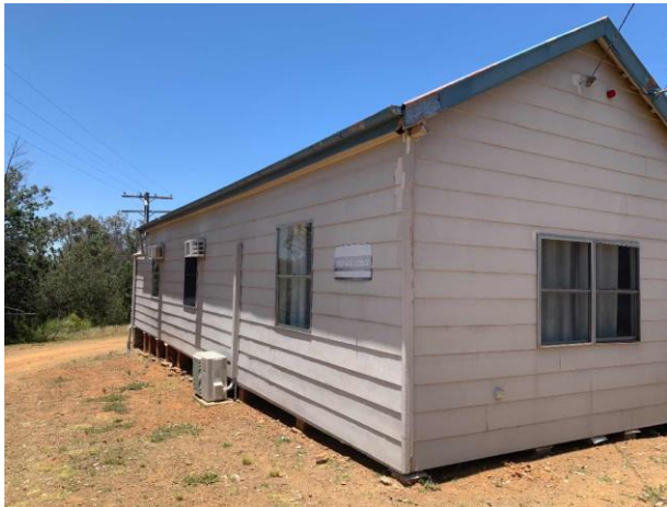
Line ID 25: External, Kilpara, Facades, Weatherboard Cladding and Joinery, Fibre Cement Sheet - Chrysotile & Amosite Asbestos Detected
