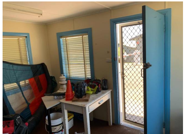
Line ID 76: Internal, Former Souvenirs Store, Throughout, Ceiling and Wall Linings, Fibre Cement Sheet - Chrysotile Asbestos Detected
