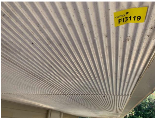
Line ID 132: External, Lodges Inc. Dilapidated Toilet B, Elevations, Underside of Awning and Trim, White Paint - Lead Detected (0.009% w/w)
