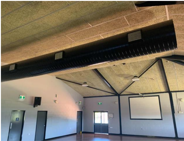
Line ID 153: Internal, Homestead, Throughout, Ceiling Space, Air Conditioning Ductwork, Insulation Material - Suspected SMF
