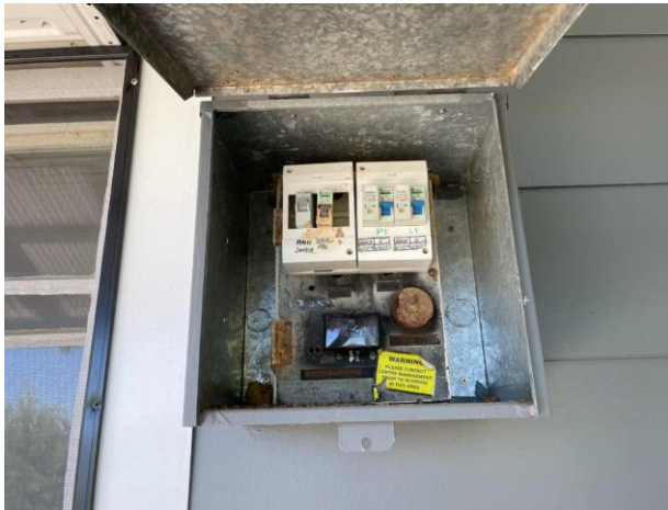
Line ID 2: External, Acacia Lodge, East and West Face, Electrical Box, Bituminous Backing Board - Suspected Asbestos
