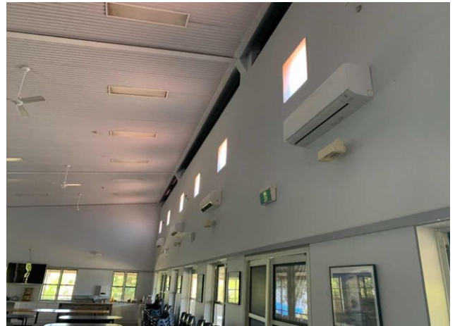
Line ID 169: Internal, Dining Hall, Throughout, Air Conditioning Units, Unknown Refrigerant - Suspected ODS
