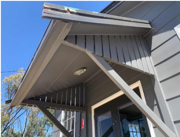
Line ID 44: External, Old Recreation Hall, South Face, Awning Lining, Fibre Cement Sheet - Chrysotile, Amosite and Crocidolite Asbestos Detected
