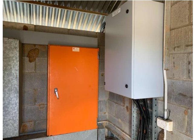
Line ID 176.1: Internal, Dining Hall, Basement, Within Closet and Roller Storage Area, Electrical Boxes - Presumed to contain asbestos or hazardous materials
