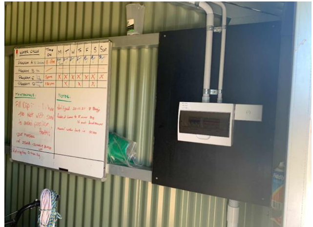
Line ID 114: Internal, Water Treatment Shed, , South Wall, Resinous Electrical Backing Board - No Asbestos Suspected
