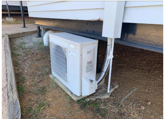
Line ID 165: External, Lodges Inc. Dilapidated Toilet B, Block C, South Elevation, Air Conditioning Units, R22 Hydrochlorofluorocarbon (HCFC) - ODS Refrigerant
