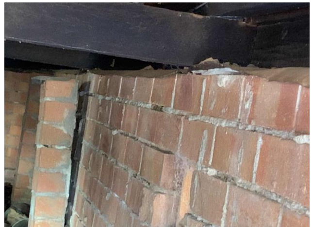
Line ID 55: External, Private Residence B, Subfloor, Column Packers, Fibre Cement Sheet - Chrysotile, Amosite and Crocidolite Asbestos Detected
