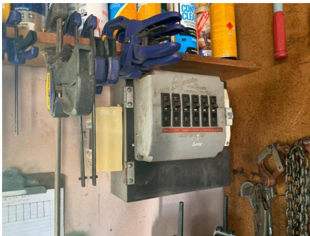
Line ID 117: Internal, Workshop, North Store, Electrical Panel, Bituminous Backing Board - Chrysotile Asbestos Detected
