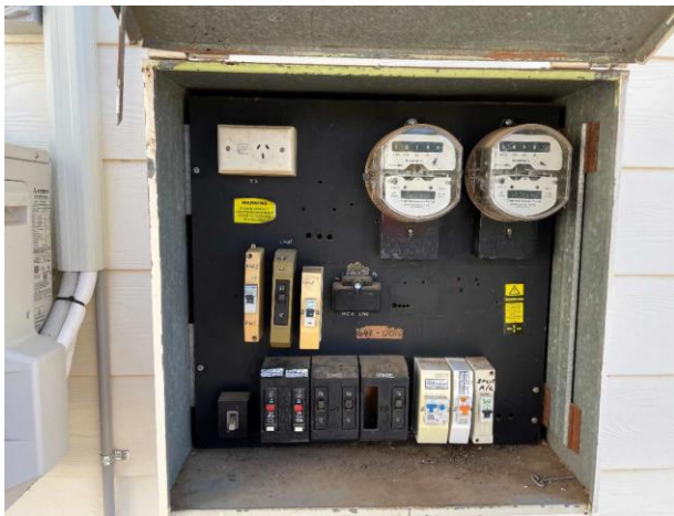
Line ID 54: External, Private Residence B, House Perimeter, Electrical Box, Bituminous Backing Board - Suspected Asbestos
