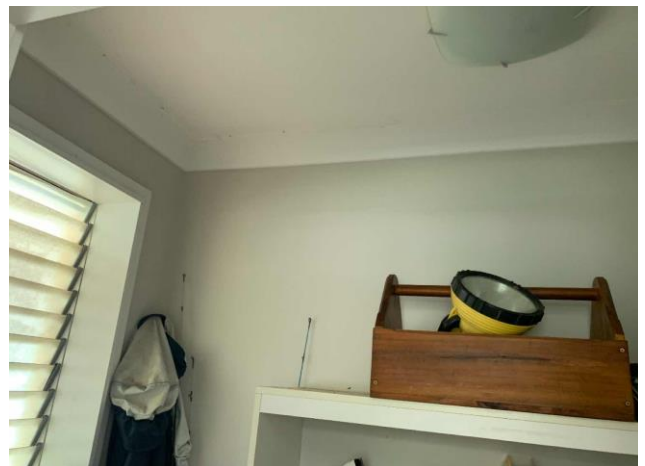
Line ID 102: Internal, Private Residence A, Laundry, Ceiling and Wall Lining, Fibre Cement Sheet - Chrysotile Asbestos Detected
