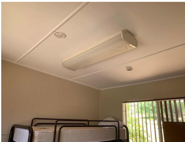
Line ID 77: Internal, Glider Complex, All Rooms, Including Toilet Areas, Walls and Ceilings, Fibre Cement Sheet - Chrysotile Asbestos Detected
