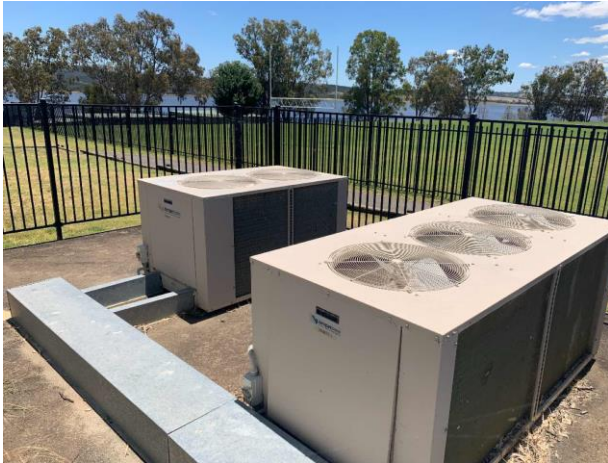
Line ID 163: External, Homestead, North Elevation, HVAC Enclosure, Condensers, Unknown Refrigerant - Suspected ODS
