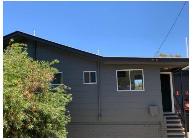
Line ID 61: External, Staff Quarters and Accommodation, Perimeter, Weatherboard Cladding and Joinery, Fibre Cement Sheet - Chrysotile & Amosite Asbestos Detected
