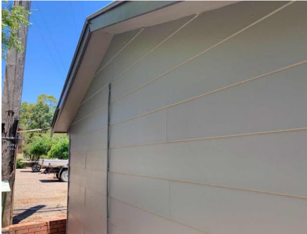
Line ID 38: External, Office, Perimeter, Eaves Lining, Fibre Cement Sheet - Chrysotile Asbestos Detected
