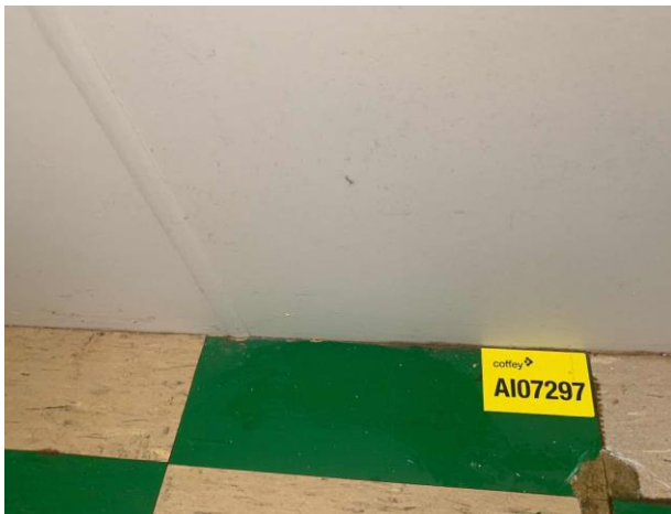
Line ID 88: Internal, Kilpara, Laundry, Floor Covering, Green Vinyl Floor Tiles - No Asbestos Detected
