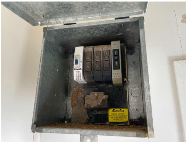
Line ID 75: Internal, Bike Shed (Formerly Male Toilet Block), On Wall, Electrical Box, Bituminous Backing Board - Suspected Asbestos
