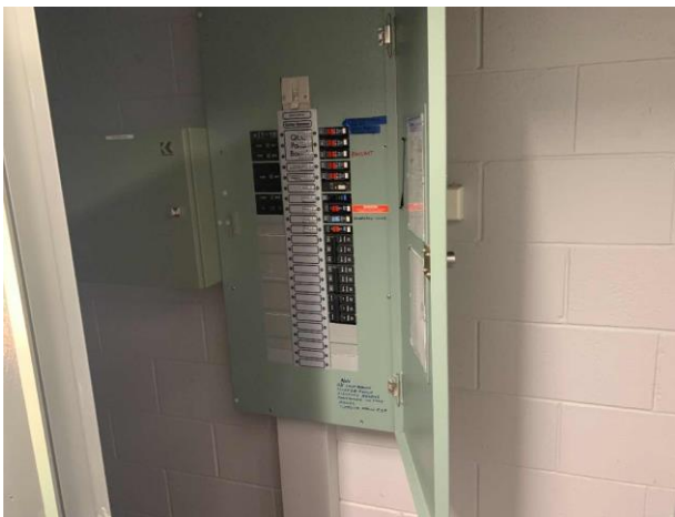
Line ID 82: Internal, Homestead, Throughout, Within Electrical Box, Bituminous Backing Board - Suspected Asbestos
