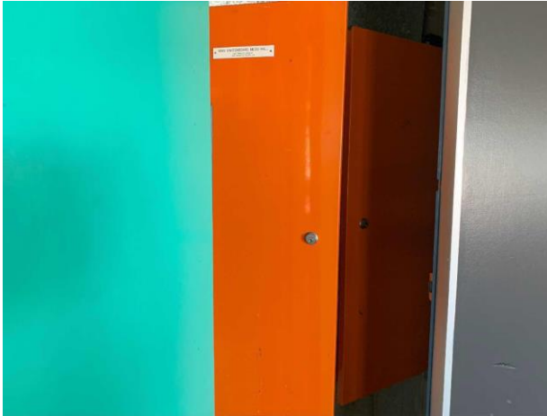
Line ID 176: Internal, Dining Hall, Basement, Within Closet and Roller Storage Area, Electrical Boxes - Presumed to contain asbestos or hazardous materials
