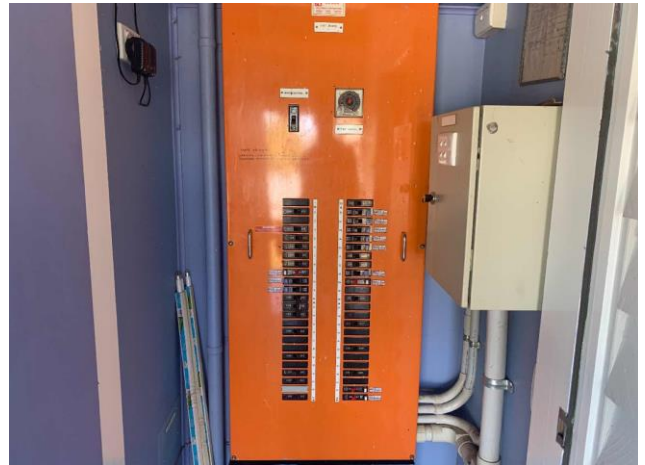
Line ID 181: Internal, Lodges Inc. Dilapidated Toilet Block, Block A, Central, Closet, Electrical Box - Presumed to contain asbestos or hazardous materials
