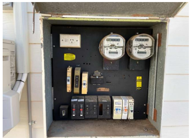
Line ID 18: External, Glider Complex, Perimeter, Electrical Box, Bituminous Backing Board - Suspected Asbestos
