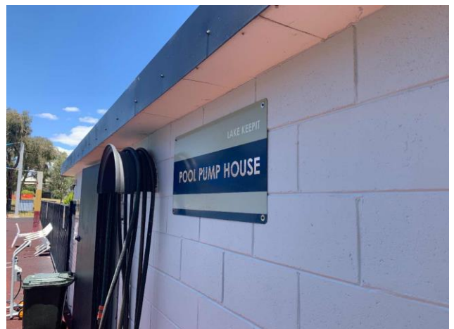
Line ID 47: External, Pool Pump House, Throughout, Eave Lining, Compressed Cement Sheet - Chrysotile, Amosite, and Crocidolite Asbestos Detected
