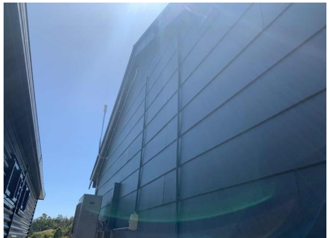
Line ID 41: External, Old (South) Dormitory, Facades, Weatherboard Cladding and Joinery, Fibre Cement Sheet - Chrysotile & Amosite Asbestos Detected
