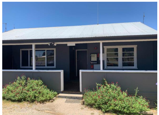
Line ID 63: External, Staff Quarters and Accommodation, Walls and Joinery, Weatherboard Cladding, Fibre Cement Sheet - Chrysotile & Amosite Asbestos Detected
