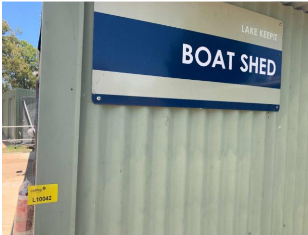
Line ID 124: External, Boat House, Throughout, Walls and Frame, Green Paint - Lead Detected (0.007% w/w)
