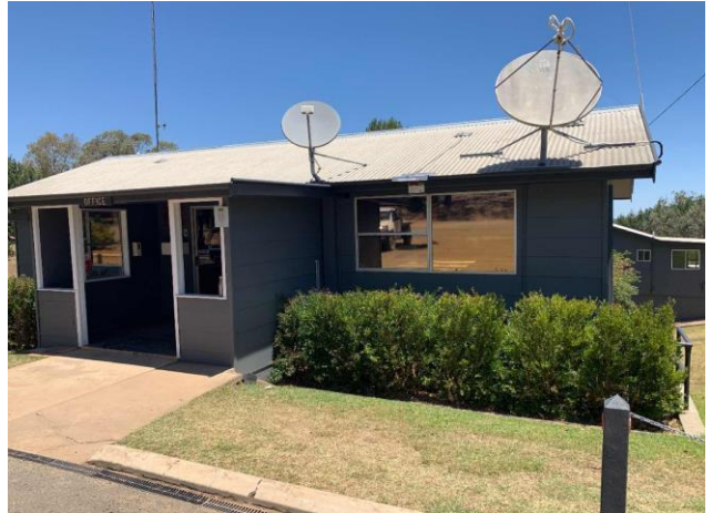
Line ID 39: External, Office, Perimeter, Weatherboard Cladding and Joinery, Fibre Cement Sheet - Chrysotile & Amosite Asbestos Detected
