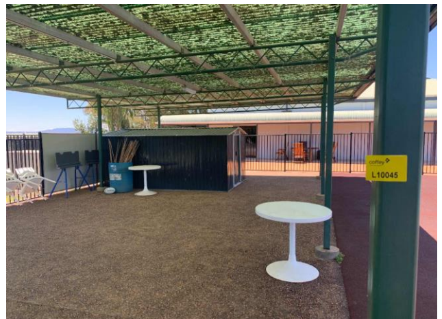
Line ID 137: External, Pool Pump House, Awning North Adjacent to Pool, Metal Frame, Coating, Green (Light) Paint - Lead Detected (0.12% w/w)
