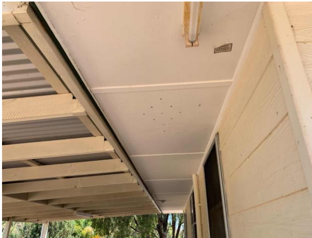
Line ID 58: External, Private Residence C, South-East Face, Awning Lining, Fibre Cement Sheet - Chrysotile, Amosite, and Crocidolite Asbestos Detected
