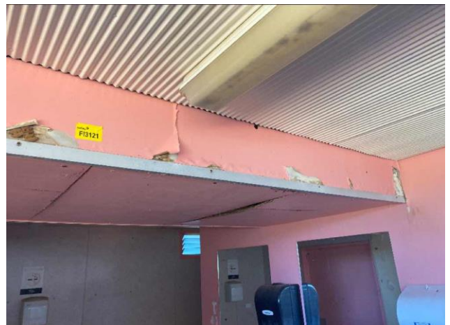
Line ID 148: Internal, Lodges Inc. Dilapidated Toilet Block, Female Toilets, Sink Walls, Pink Paint - Lead Detected (0.02% w/w)
