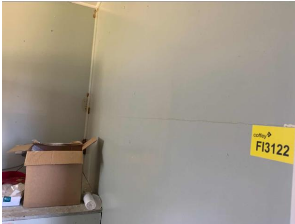
Line ID 145: Internal, Lodges Inc. Dilapidated Toilet Block, Block B, Basement, Laundry Room, Walls, Light Blue Paint - Lead Detected (<0.005% w/w)
