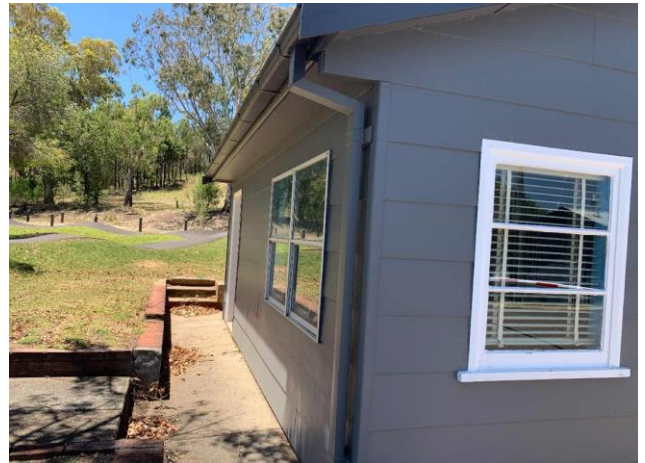
Line ID 14: External, Former Souvenirs Store, Facades, Weatherboard Cladding and Joinery, Fibre Cement Sheet - Chrysotile & Amosite Asbestos Detected
