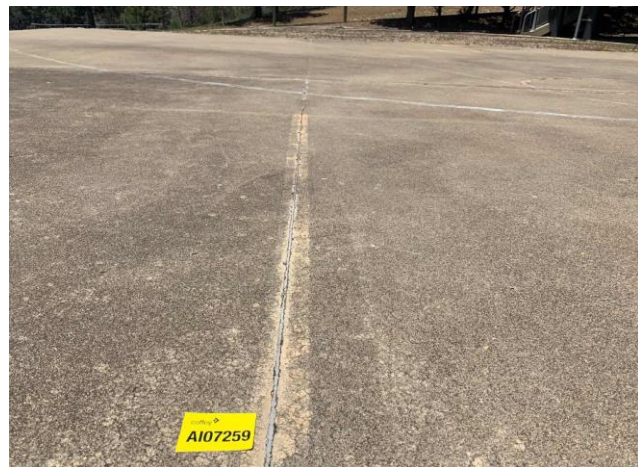
Line ID 12: External, Dining Hall, Throughout, North, Adjacent Concrete Sporting Pad, Expansion Joints, Construction Joint Mastic - No Asbestos Detected
