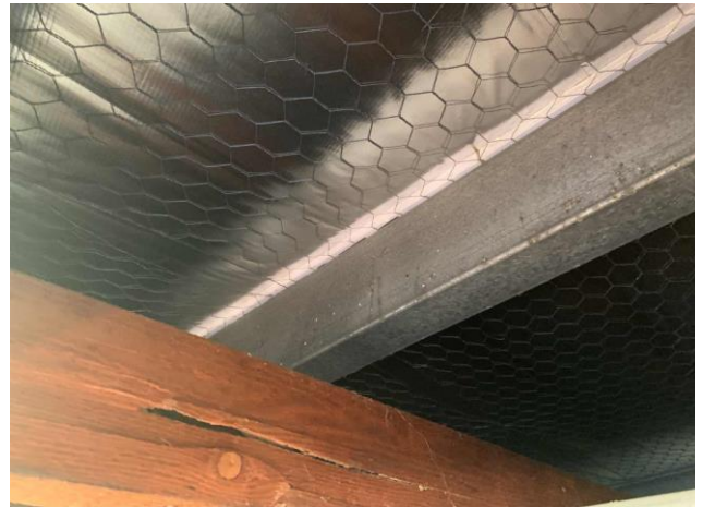
Line ID 160: Internal, Lodges Inc. Dilapidated Toilet Block, Male Toilets, Ceiling Space, Underside of Roof, Sarking Insulation - Suspected SMF
