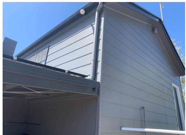
Line ID 98: Internal, Old Recreation Hall, North Extension (Between NE & SE Rooms), Weatherboard Cladding and Joinery, Fibre Cement Sheet - Chrysotile & Amosite Asbestos Detected
