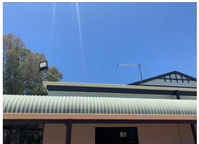
Line ID 24: External, Homestead, Roof, Build-out Panelling, Compressed Cement Sheet - Suspected Asbestos
