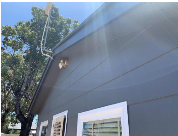
Line ID 15: External, Former Souvenirs Store, Perimeter, Eaves Lining, Fibre Cement Sheet - Chrysotile Asbestos Detected
