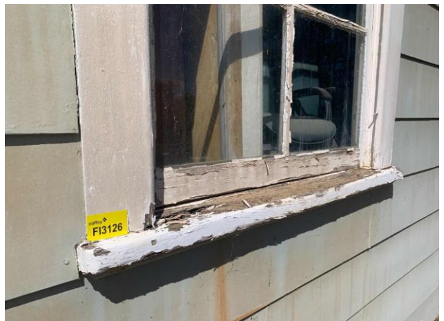
Line ID 128: External, Hilltop Lodge, Elevations, East Elevation, Window Frames, White Paint - Lead Detected (0.03% w/w)
