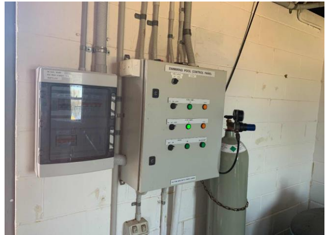
Line ID 100: Internal, Pool Pump House, North Wall, Within Electrical Box, Resinous Electrical Backing Board - Suspected Asbestos
