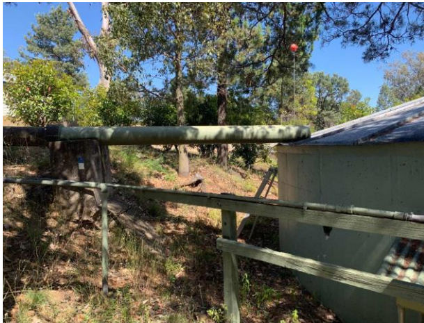
Line ID 6: External, Archery Range, Water Tank Area, Tank Adjacent Road, Pipework, Moulded Fibre Cement - Chrysotile, Amosite and Crocidolite Asbestos Detected
