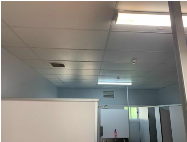
Line ID 159: Internal, Lodges Inc. Dilapidated Toilet Block, Block C, Toilets and Shower Area, Ceilings, Compressed Ceiling Tiles - Suspected SMF
