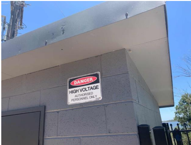
Line ID 13: External, Electrical Substation on Access Road to Kilpara, Perimeter, Eaves Lining, Fibre Cement Sheet - Chrysotile Asbestos Detected
