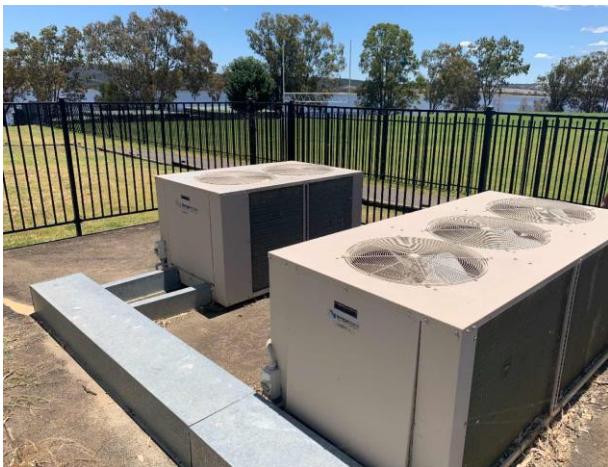
Line ID 166: External, Pool Pump House, Awning North Adjacent to Pool, HVAC Enclosure, Compressor Units, Unknown Refrigerant - Suspected ODS
