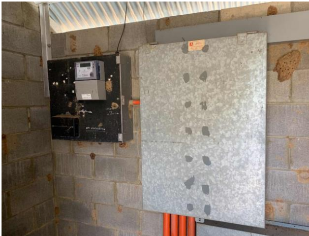
Line ID 176.2: Internal, Dining Hall, Basement, Within Closet and Roller Storage Area, Electrical Boxes - Presumed to contain asbestos or hazardous materials
