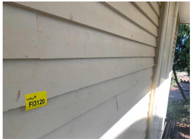
Line ID 131: External, Lodges Inc. Dilapidated Toilet B, Elevations, Fascia, Cream Paint - Lead Detected (<0.005% w/w)
