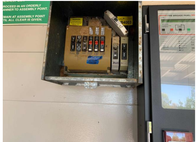
Line ID 26: External, Kilpara, North Wall, Electrical Cabinet, Bituminous Backing Board - Chrysotile Asbestos Detected
