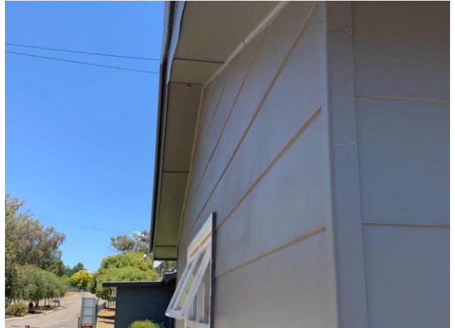
Line ID 66: External, Workshop, Perimeter, Eaves Lining, Fibre Cement Sheet - Chrysotile Asbestos Detected
