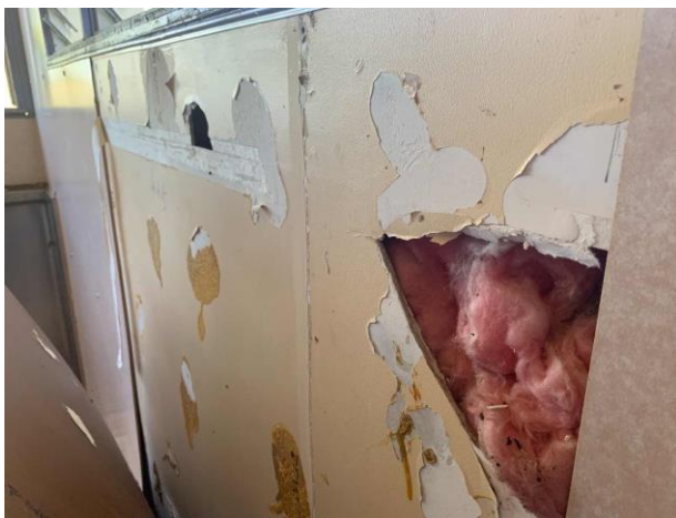
Line ID 161: Internal, Lodges Inc. Dilapidated Toilet Block, Male Toilets, Within Walls, Insulation Batt's - Suspected SMF
