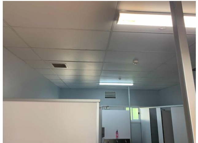
Line ID 158: Internal, Lodges Inc. Dilapidated Toilet Block, Block B, Toilets and Shower Area, Ceilings, Compressed Ceiling Tiles - Suspected SMF
