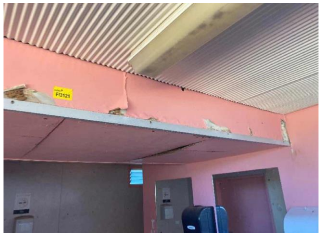
Line ID 91: Internal, Lodges Inc. Dilapidated Toilet Block, Female Toilets, Walls Throughout, Compressed Cement Sheet - No Asbestos Detected
