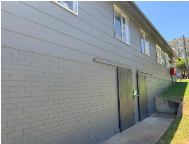
Line ID 67: External, Workshop, Perimeter, Weatherboard Cladding and Joinery, Fibre Cement Sheet - Chrysotile & Amosite Asbestos Detected
