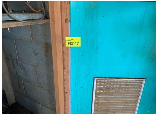
Line ID 142: Internal, Dining Hall, Basement, Within Closets, Timber Trim and Doors, Teal Paint - Lead Detected (<0.005% w/w)
