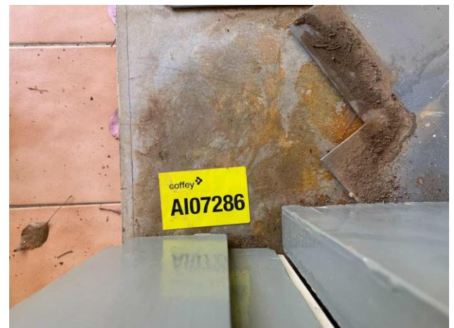
Line ID 78: Internal, Glider Complex, Laundry, Below Vinyl Floor Tiles, Compressed Cement Sheet - Chrysotile Asbestos Detected
