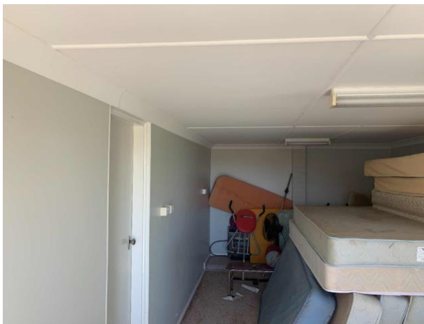
Line ID 101: Internal, Private Residence A, Basement Room, Ceiling Lining, Fibre Cement Sheet - Chrysotile, Amosite and Crocidolite Asbestos Detected
