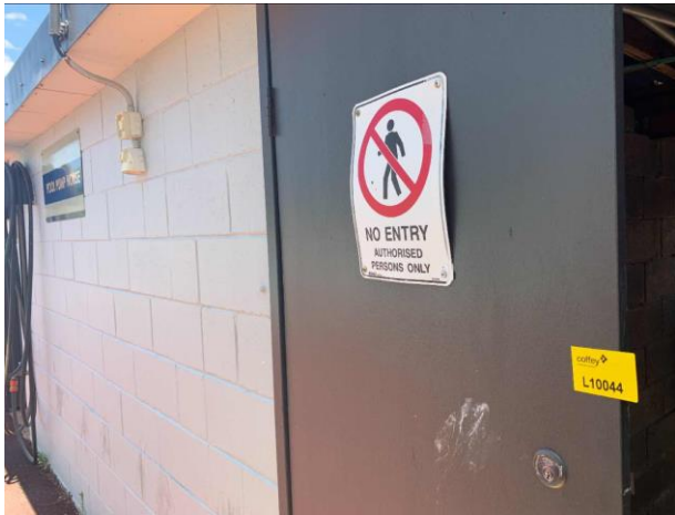
Line ID 138: External, Pool Pump House, Throughout, Doors, Door Frames and Trim, Grey Paint - Lead Detected (<0.005% w/w)
