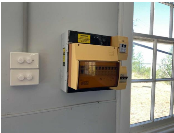
Line ID 97: Internal, Old Recreation Hall, North Extension (Between NE & SE Rooms), Electrical Box, Bituminous Backing Board - Suspected Asbestos
