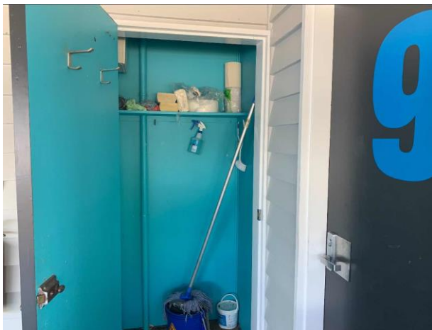
Line ID 147: Internal, Lodges Inc. Dilapidated Toilet Block, Block C, Utility Closets Throughout, Teal Paint - Lead Detected (<0.005% w/w)
