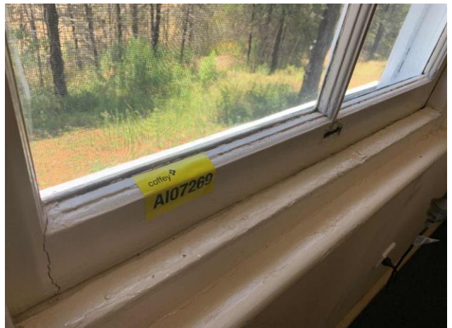
Line ID 70: Internal, Acacia Lodge, Kitchen Lodge, Windows Between Pane and Frame, Mastic Material - No Asbestos Detected
