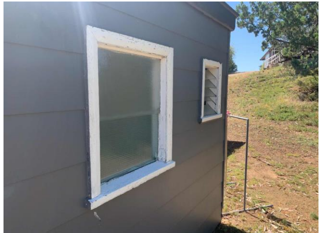
Line ID 123: External, Bike Shed (Formerly Male Toilet Block), Elevations, Trim work Throughout, White Paint - Lead Detected (0.6% w/w)
