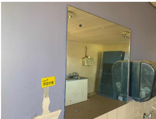
Line ID 149: Internal, Lodges Inc. Dilapidated Toilet Block, Male Toilets, Walls and Trim, Purple Paint - Lead Detected (0.03% w/w)
