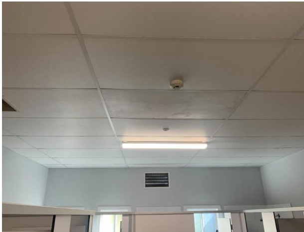
Line ID 157: Internal, Lodges Inc. Dilapidated Toilet Block, Block A, Toilets and Shower Area, Ceiling, Compressed Ceiling Tiles - Suspected SMF
