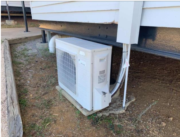
Line ID 164.1: External, Lodges Inc. Dilapidated Toilet B, Elevations, North, Air Conditioning Unit, R22 Hydrochlorofluorocarbon (HCFC) - ODS Refrigerant
